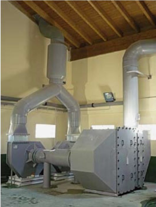
Deodorization by Compact Active Carbon Equipment with dual stage, Q=9,200 m 3 /h.
